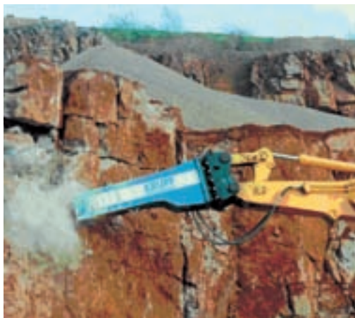
Photo B: closely-spaced discontinuities are necessary to excavate in-situ rock with an impact hammer
